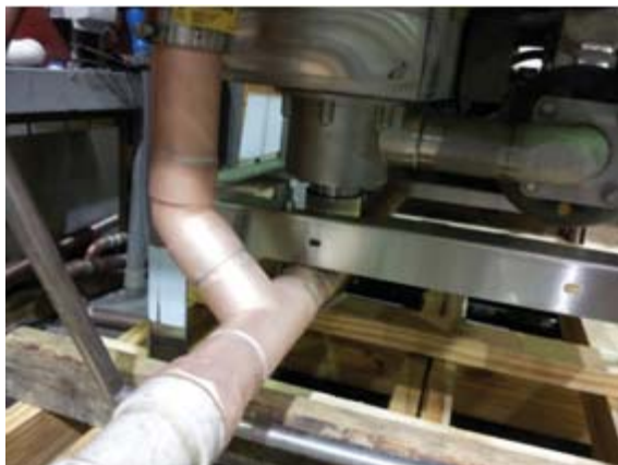
Showing 2" drain manifold exiting sump & scrap box
