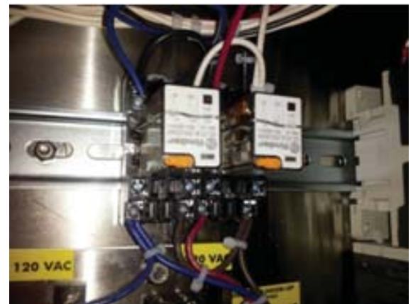
Conveyor motor control relays
