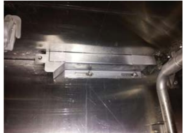
Diverter plate separates fill stream for wash and rinse tank
