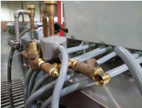
Hot water inlet manifold, single point 3/4" pipe, PR valve
