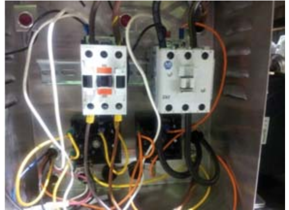
T-stat signal goes to term #6 on heater relay under contactor
