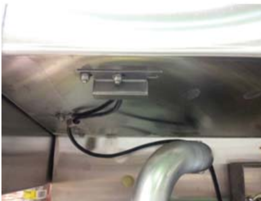
Sequence reed switch for wash tank
