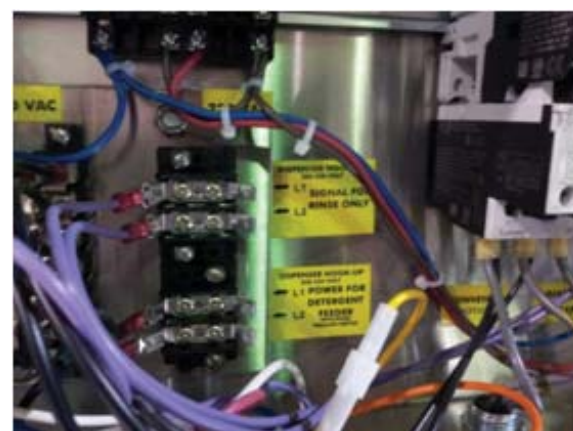
Dispenser signal connection terminals in control box
