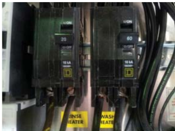
Rinse and wash heater circuit breakers in the control box
