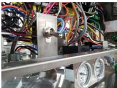
De-lime switch in HT25 control box
