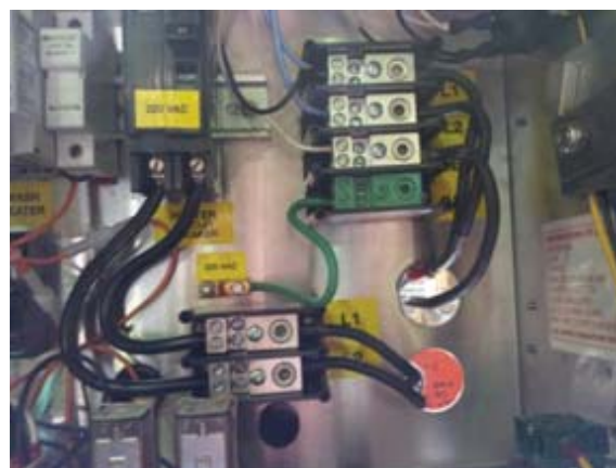
Main distribution blocks for two incoming circuits, 30/60a
