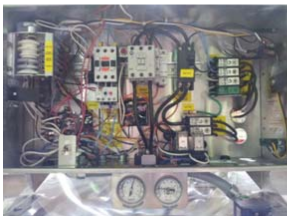
Showing HT-25, single-phase control box
