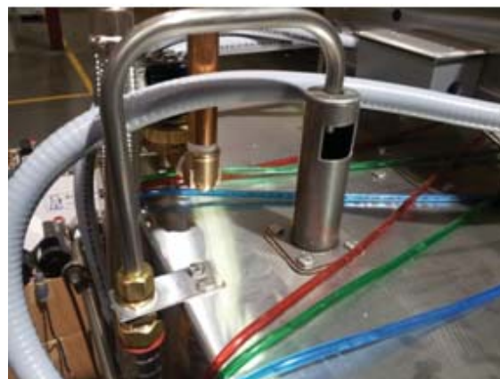
Connection from bkr to heater ~ from heater to air-gap
