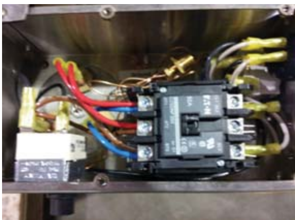
Showing hi-limit switch at left of contactor
