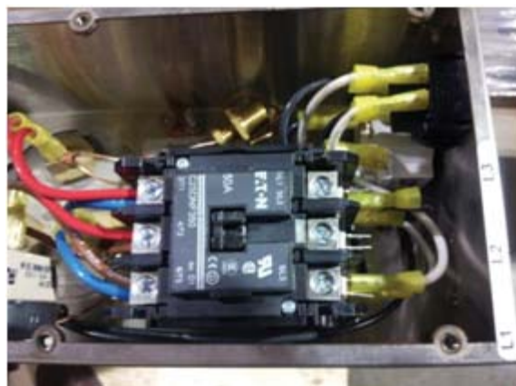
Connection point for wires on right-side of contactor
