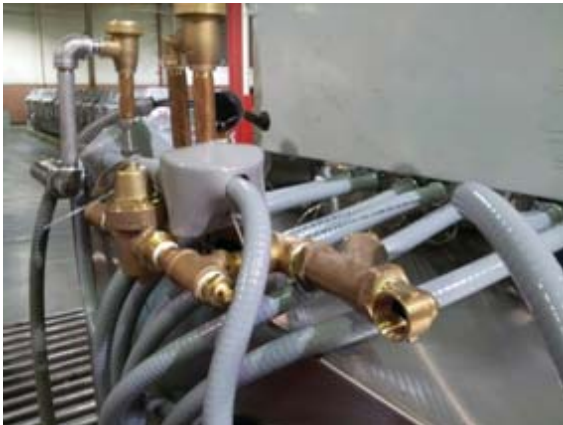
Hot water inlet manifold, single point 3/4" pipe, PR valve
