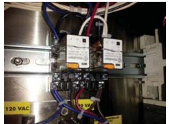
Conveyor motor control relays
