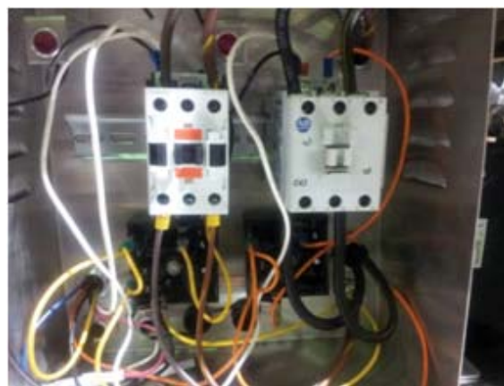
Showing heater contactors with heater relays underneath
