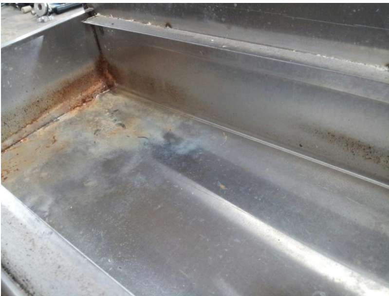
(Showing rusting above the water)
