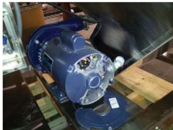
66 power scrapper motor, 1.5 HP, 208v, single-phase
