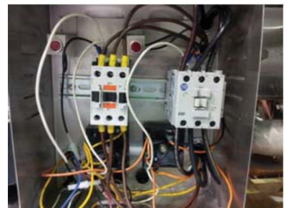
T-stat signal goes to term #6 on heater relay under contactor
