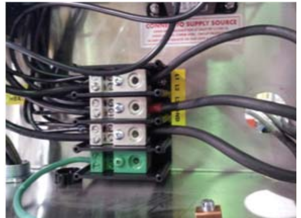
Main distribution block for 44's incoming 3-phase
