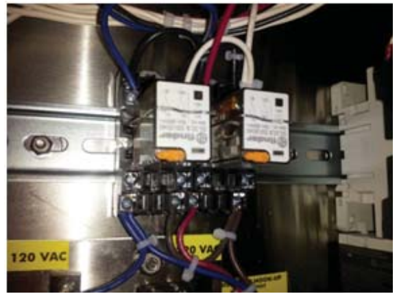
Conveyor motor control relays
