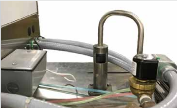
Showing 1/2" female pipe inlet, ball valve, y-line filter, water solenoid, ASSE approved air gap (backflow preventer)
