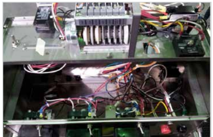
Showing AWS control tray lifted to service pumps
