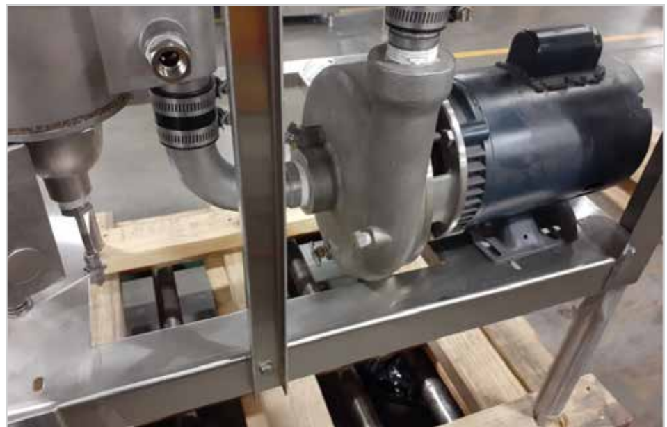
Wash Pump and Motor
