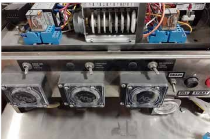
Showing AWS-H control tray in normal position
