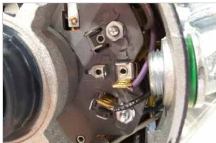
Line connection spades for L1, Neu (arrow 1 & 2)
